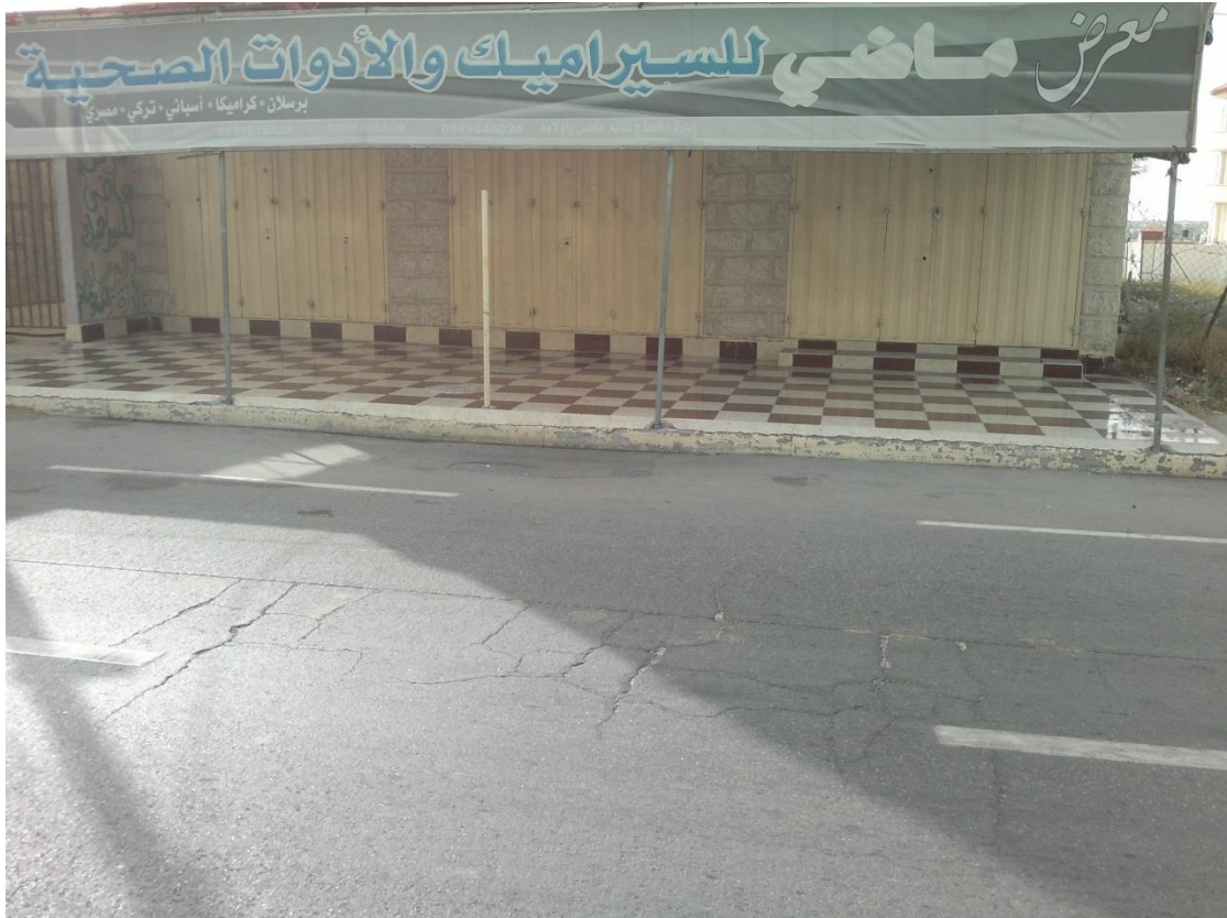
Figure (3.5): Omar Ibn Al-Khattab street distresses.
