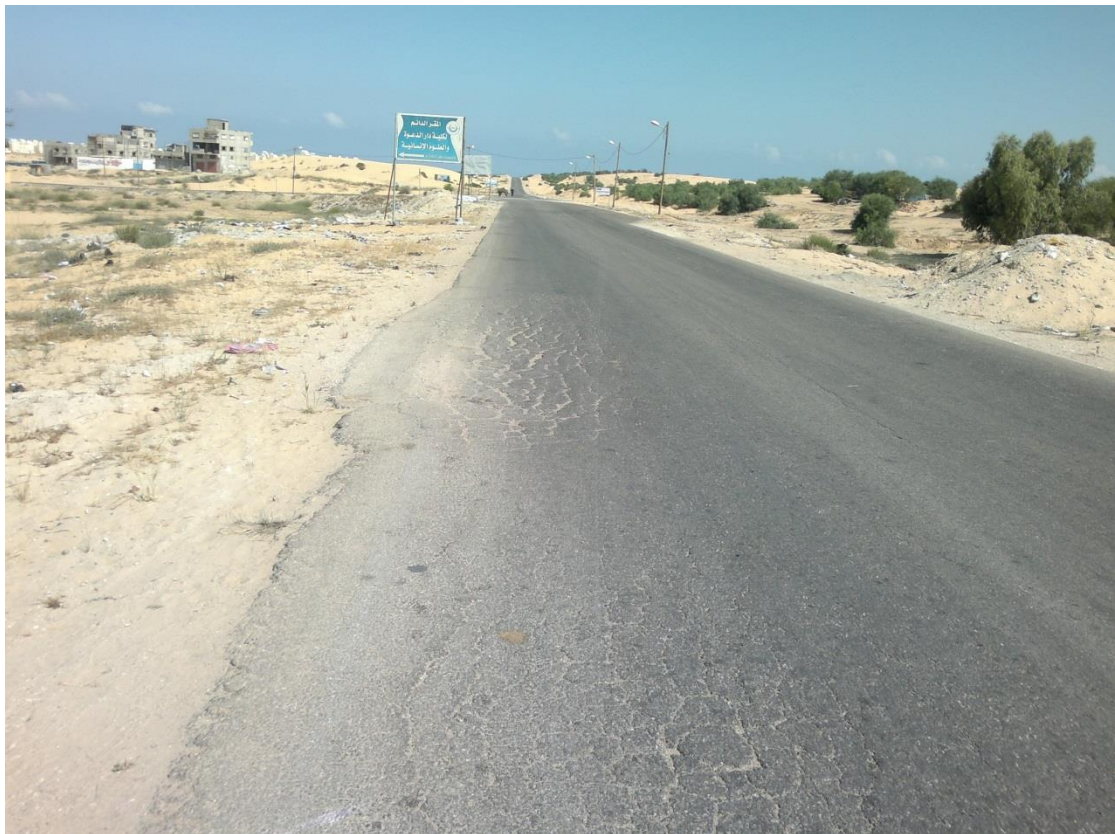
Figure (3.6): Moraj street distresses.
