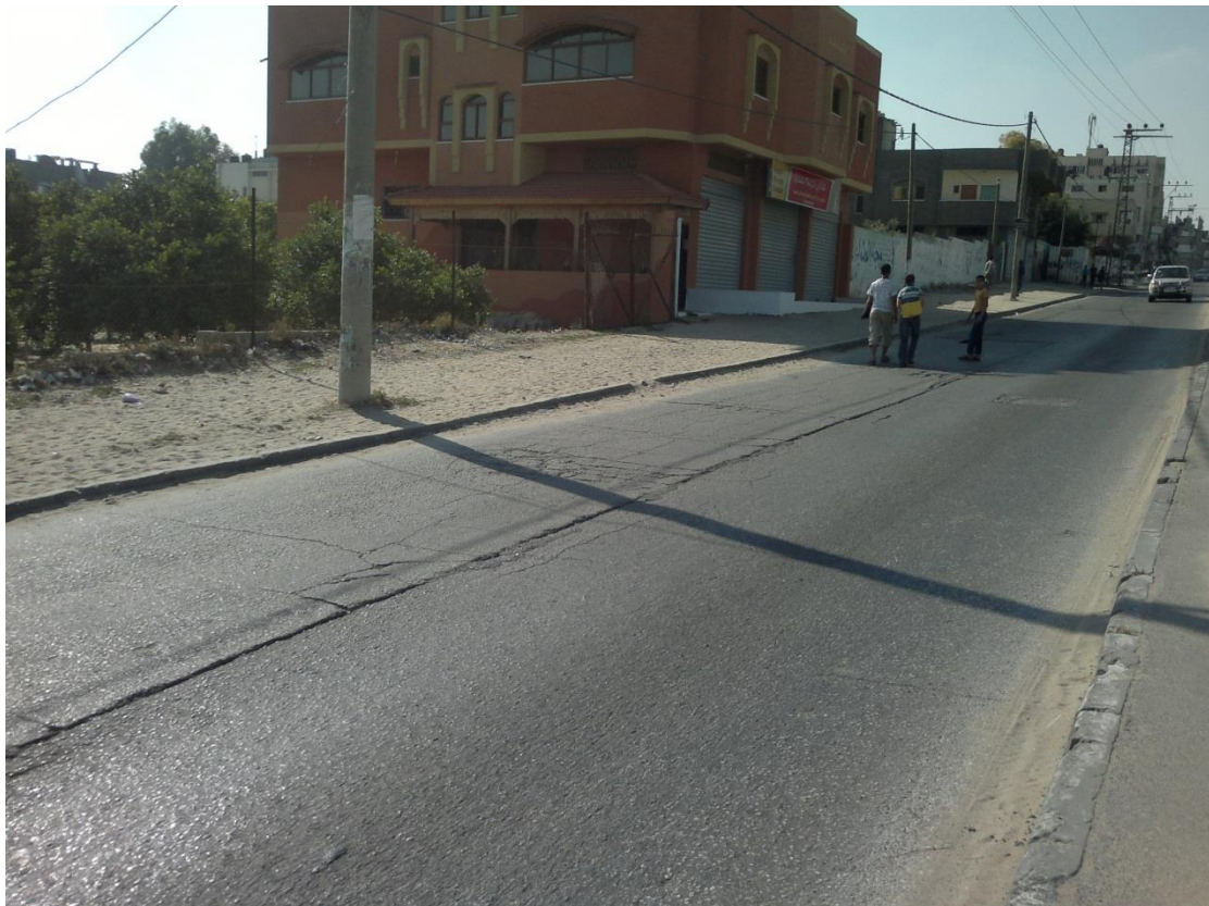
Figure (3.8): Abu Baker El-Seddeq street distresses.
